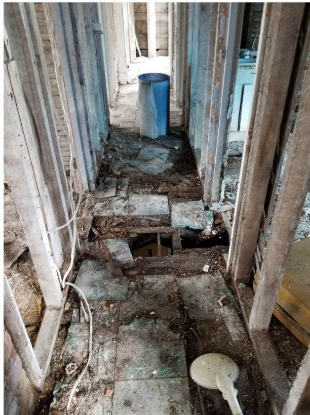
18. Second floor –floor damaged for fighting fire
