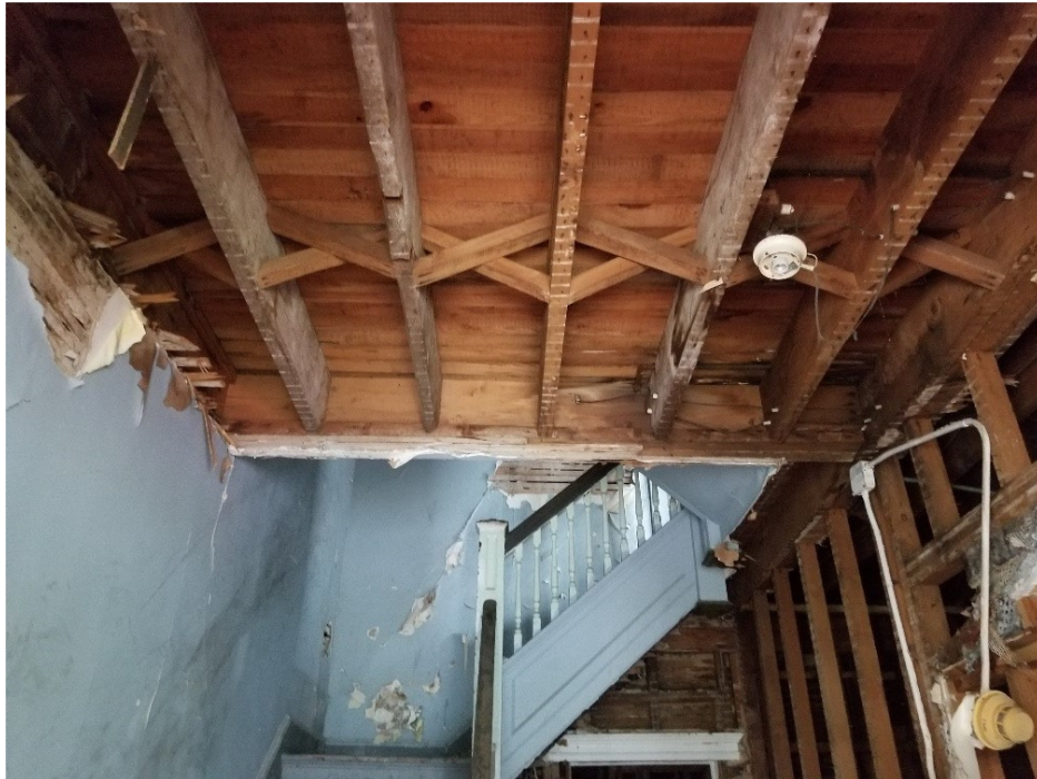
22. First floor –Stairs from the Second floor and ceiling framing still intact.
