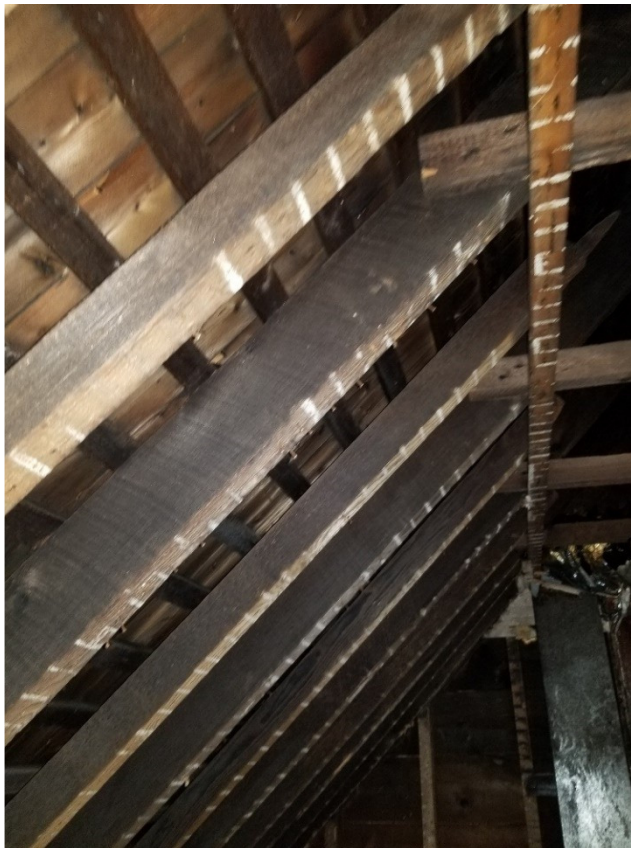
11 and 12. Attic floor –Roof rafters still intact. Roof sheathing charred.
