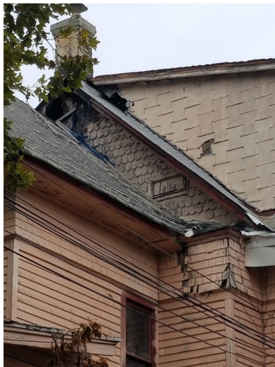
4. Exterior view –Façade siding and Fire damage
