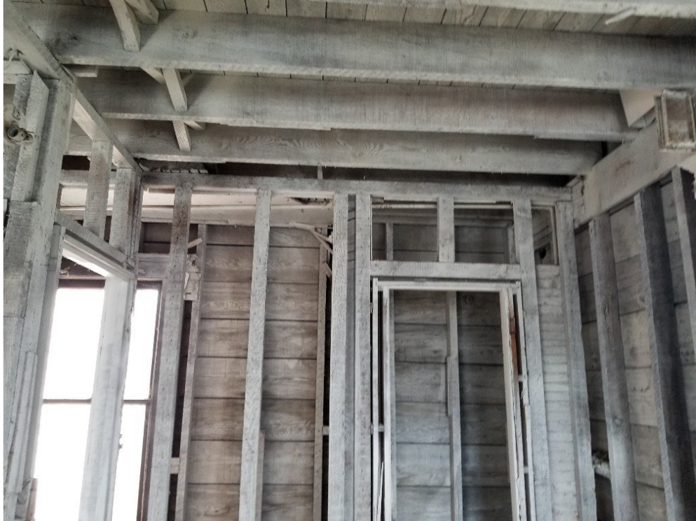
17. Second floor –Ceiling joists, Interior and exterior framing still intact.
