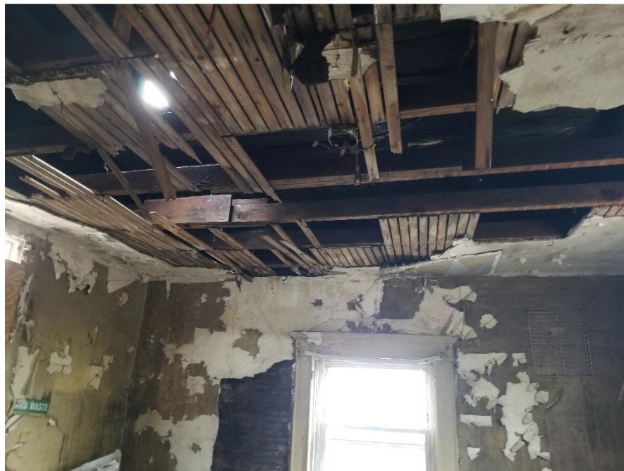
10. Attic floor –Fire damage to roof rafters, partitions still intact
