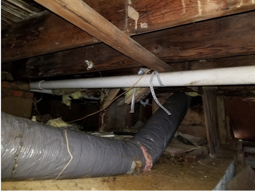
27. Cellar -Crawl space. Floor framing still intact.
