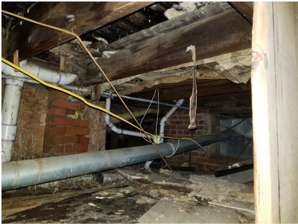
28. Cellar -Crawl space. Floor framing still intact.
