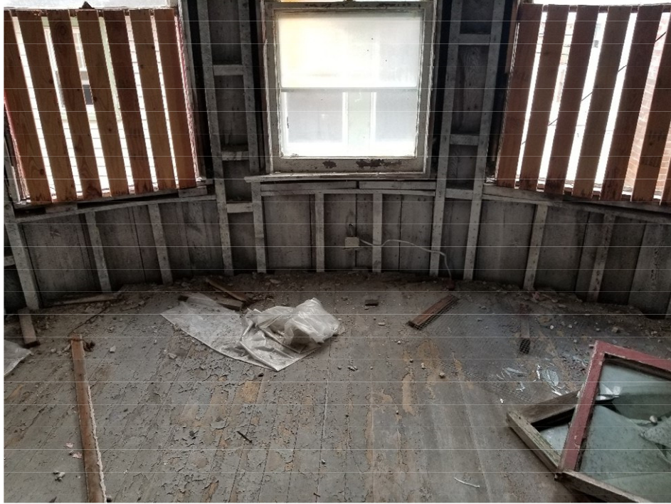
19. Second floor – Exterior framing and floor still intact.
