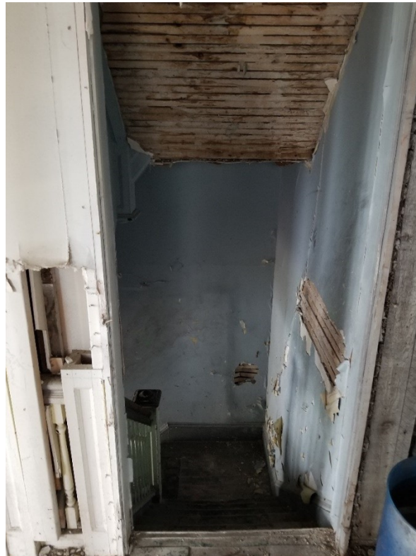
14. Second floor –Stairs down to First floor still intact.
