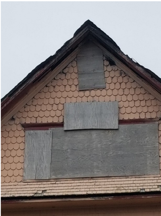
3. Exterior view –Façade siding and Fire damage
