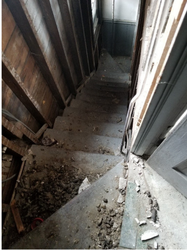
15. Second floor –Rear stairs down to First floor still intact.
