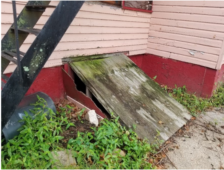
8. Exterior view –Missing Bilco door
