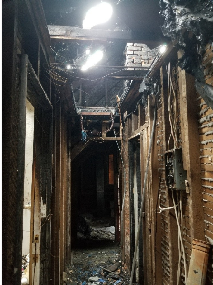
9. Attic floor –Fire damage to roof rafters, partitions still intact
