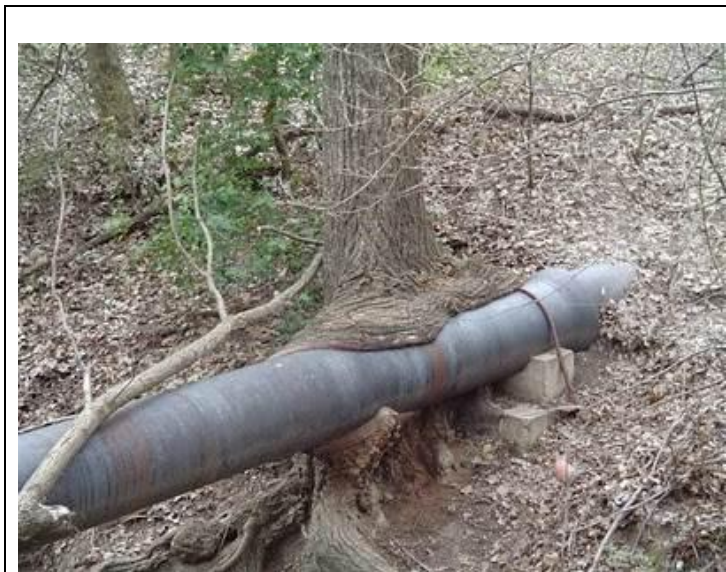
Image 1: There is little to no lateral movement that can be observed in this pipe even though there is no support from soil on the other side of the tree.
