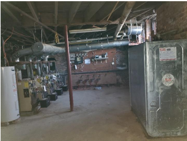
Image 3. Fuel oil tank, pump, and filter system in the basement boiler room
