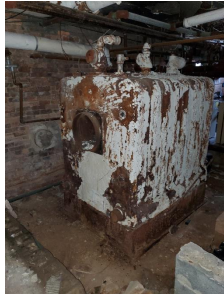
Image 4. Steam Condensate System in the basement boiler room
