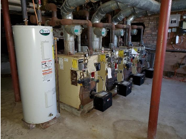
Image 1. Front view of boilers in basement boiler room
