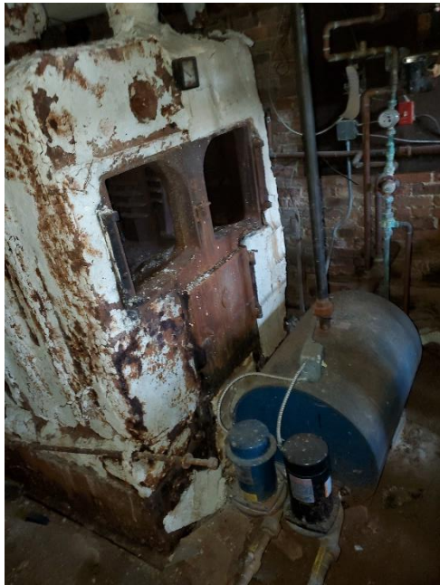
Image 5. Steam Condensate System in the basement boiler room
