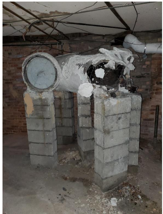
Image 6. Boiler Room steam pipe
