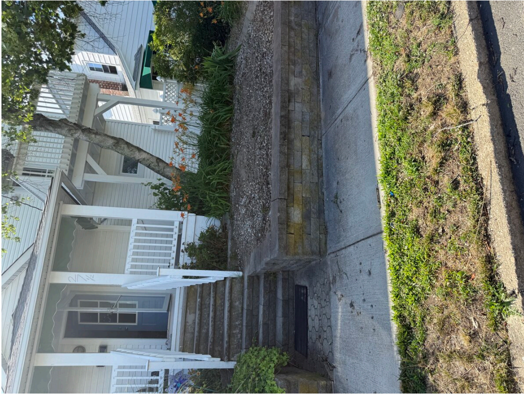
Figure 1: Front yard of subject property showing elevated grade, retaining wall, and proximity to sidewalk.
